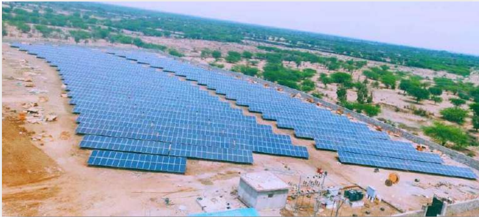
933 kW Captive Solar Plant at Bhilwara, Rajasthan
