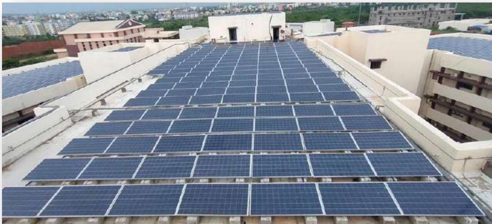
1.2 MW Rooftop Solar Plant at Bhubaneswar, Odisha
